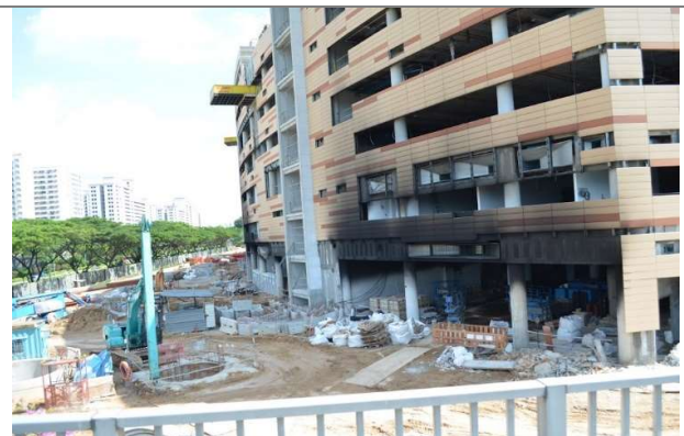
Fire damage to building under construction
